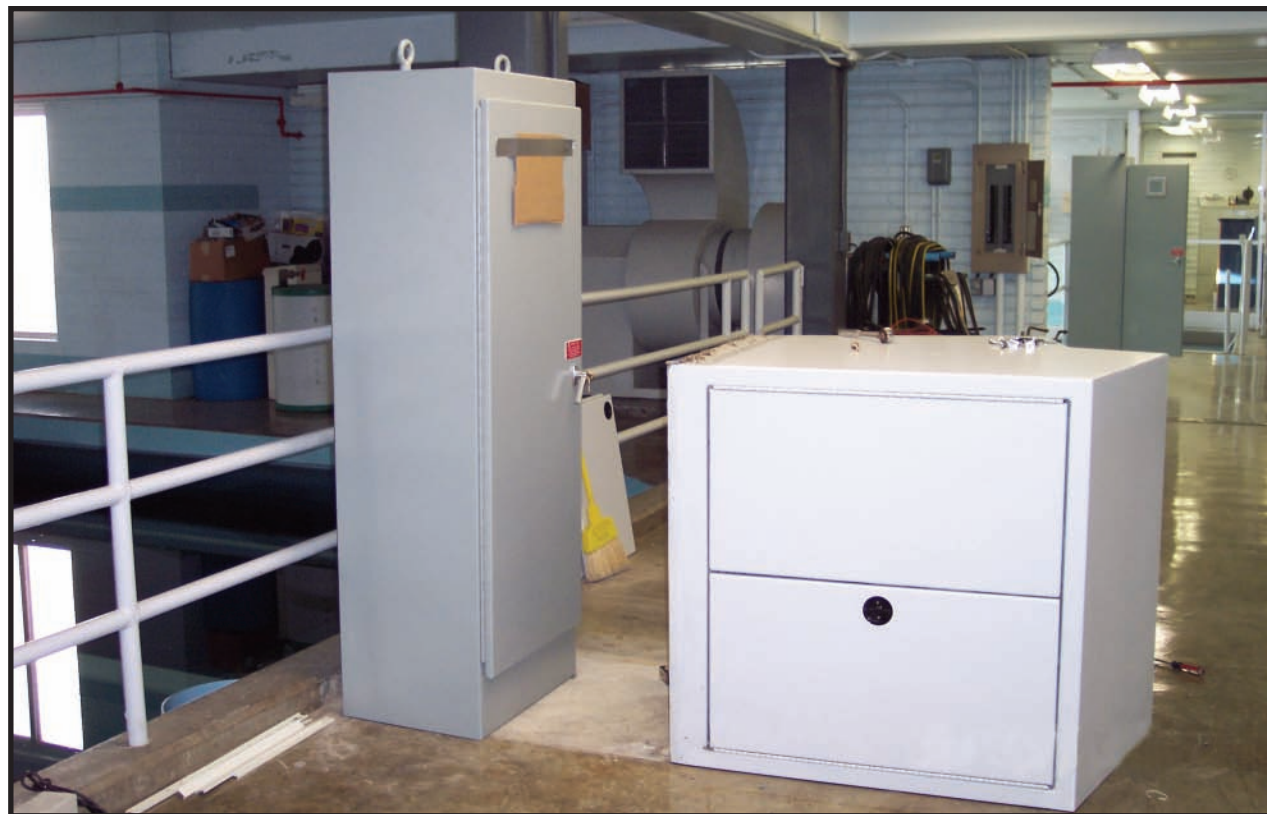
New computerized filter consoles with touch screens and ethernet to main computers replacing pneumatic controls and manually operated valves.
